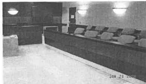
4. Courtroom 103, wood base removed at jury Wall.
