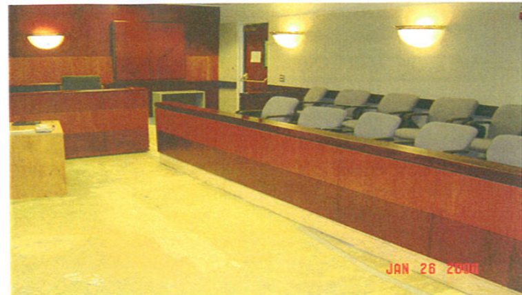
4. Courtroom 103, wood base removed at Jury Wall.
