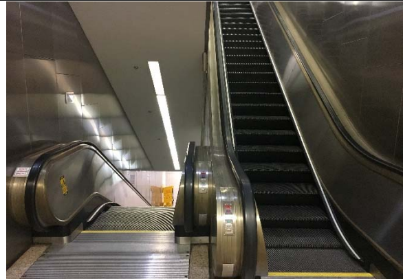
Stanley Mosk Courthouse - LA - Escalators Phase 2
