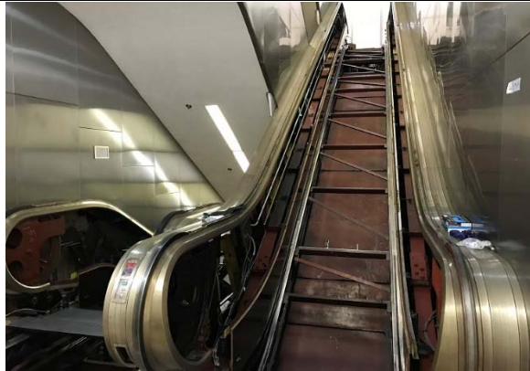
Stanley Mosk Courthouse - LA - Escalators Phase 2
