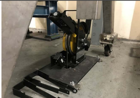
Edelman Children's Court - LA - Elevator
