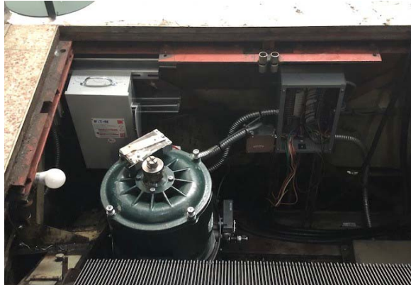
Stanley Mosk Courthouse - LA - Escalators Phase 4
