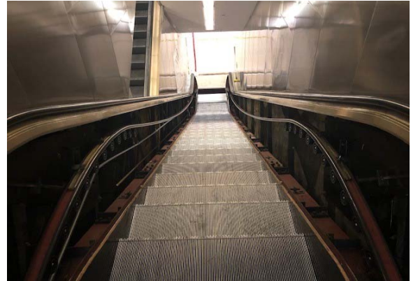
Stanley Mosk Courthouse - LA - Escalators Phase 4
