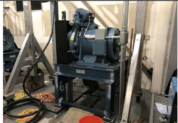
Edelman Children's Court - LA - Elevator
