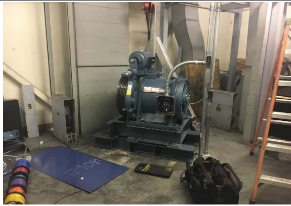
Alhambra Courthouse - LA - Elevator
