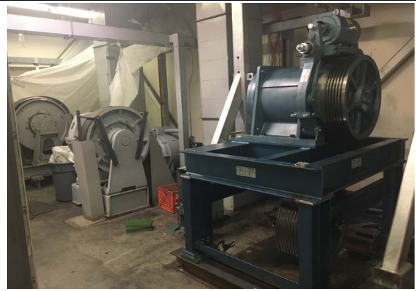
Alhambra Courthouse - LA - Elevator
