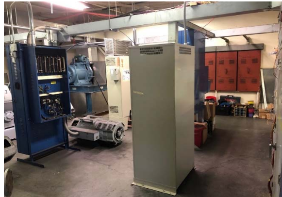
Alhambra Courthouse - LA - Elevator
