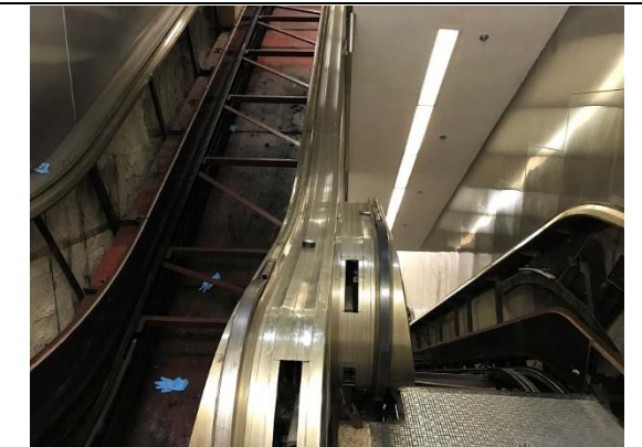
Stanley Mosk Courthouse - LA - Escalators Phase 5
