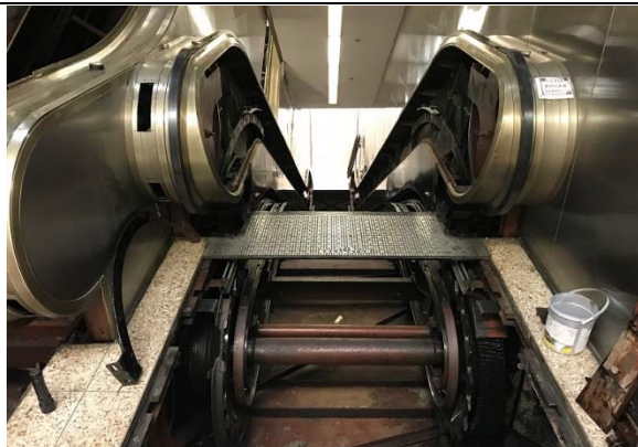
Stanley Mosk Courthouse - LA - Escalators Phase 5
