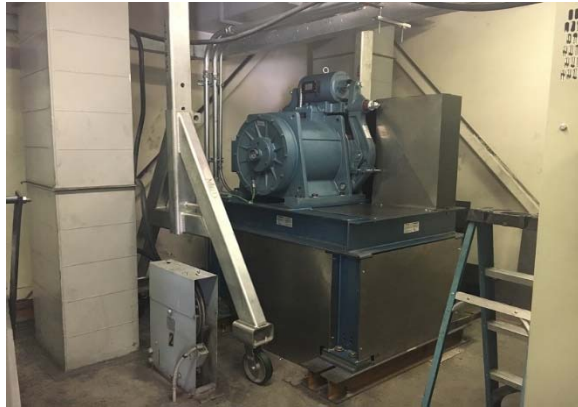
Alhambra Courthouse - LA - Elevator
