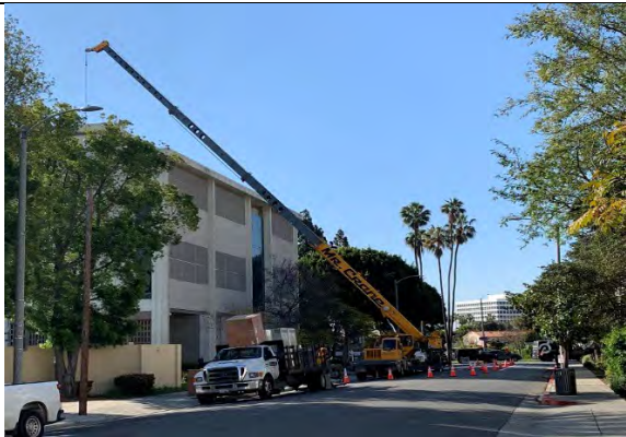
Beverly Hills - LA - Elevator
