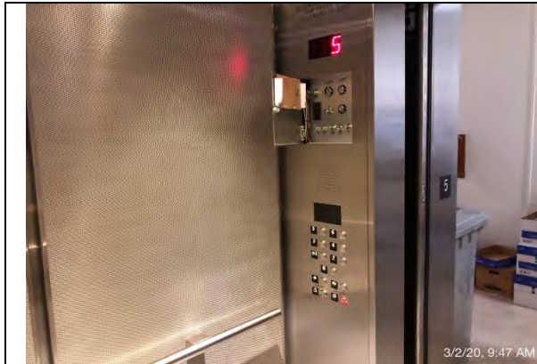
Inglewood Courthouse - LA - Elevator
