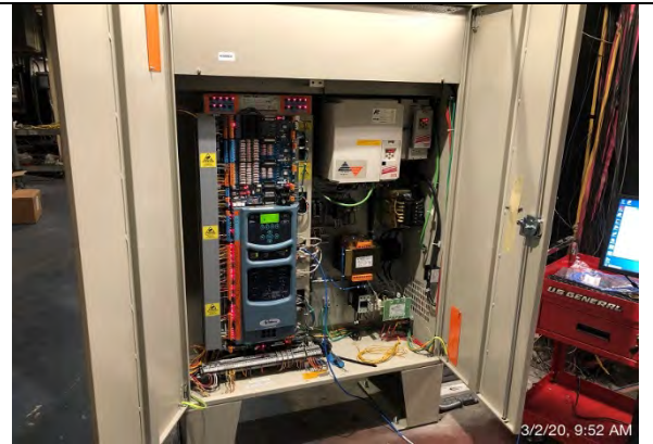
Inglewood Courthouse - LA - Elevator
