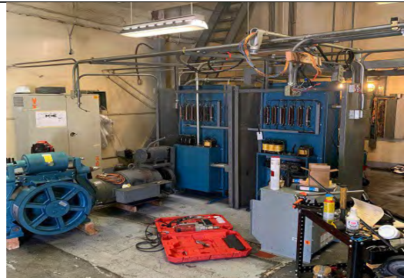
Beverly Hills - LA - Elevator
