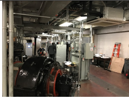
Stanley Mosk Courthouse Elevator Machine Room - After
