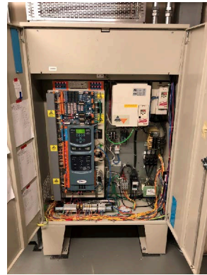
Edelman Courthouse – New Controller
