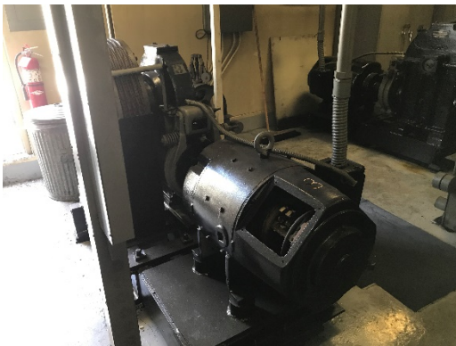
Beverly Hills Courthouse – Elevators #3 & #4 Old Machines
