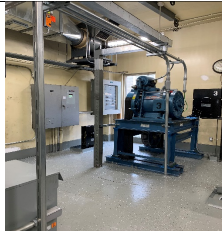
Beverly Hills Courthouse – Elevators #3 & #4 New Machines
