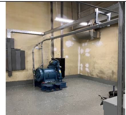
Beverly Hills Courthouse – Elevators #1 New Machine
