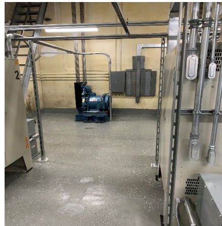
Beverly Hills Courthouse – Elevators #2 New Machine
