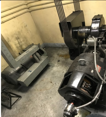
Beverly Hills Courthouse – Elevators #2 Old Machine
