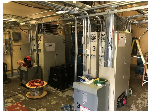
Beverly Hills Courthouse – New Elevators Controllers
