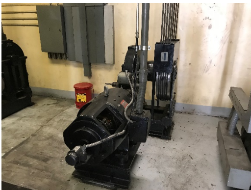
Beverly Hills Courthouse – Elevators #1 Old Machine
