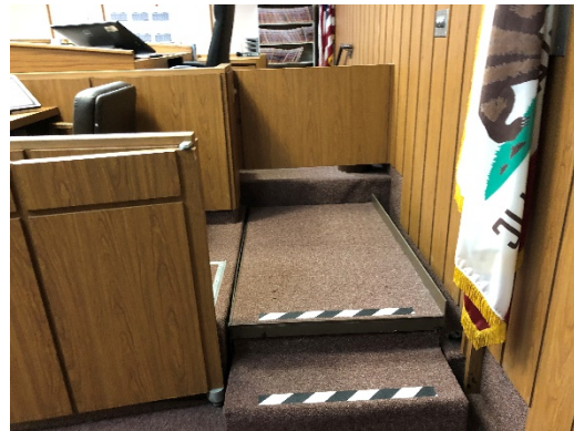
Downey Courthouse – Refurbished Wheelchair lift
