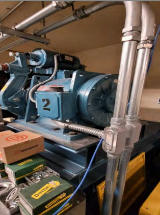
El Monte Courthouse – Elevator 2 New Hoist Machine
