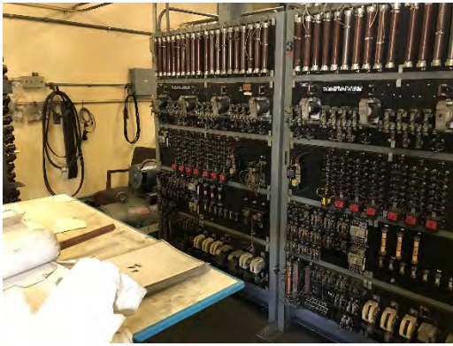
Beverly Hills Courthouse – Old Elevators Controllers
