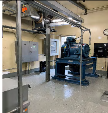
Beverly Hills Courthouse – Elevators #3 & #4 New Machines
