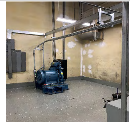
Beverly Hills Courthouse – Elevators #1 New Machine
