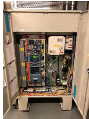
Edelman Courthouse – New Controller
