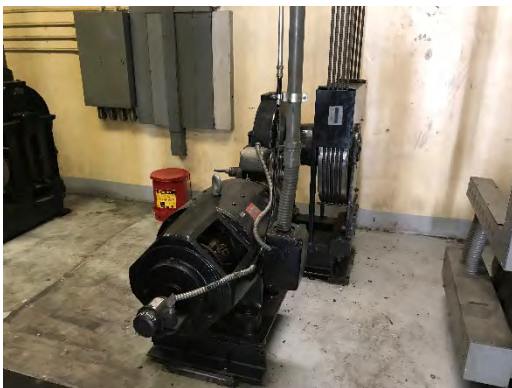
Beverly Hills Courthouse – Elevators #1 Old Machine
