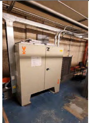
El Monte Courthouse – Elevator 2 New Controller
