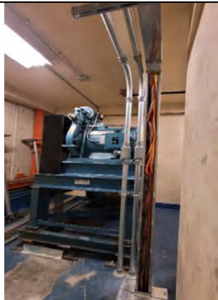
El Monte Courthouse – Elevator 5 New Hoist Machine
