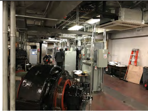
Stanley Mosk Courthouse Elevator Machine Room - After
