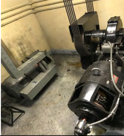
Beverly Hills Courthouse – Elevators #2 Old Machine
