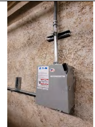
El Monte Courthouse – Elevator 2 New
