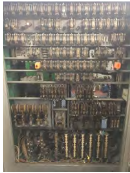
Torrance Courthouse – Old Controller
