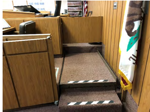
Downey Courthouse – Refurbished Wheelchair lift
