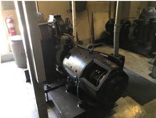
Beverly Hills Courthouse – Elevators #3 & #4 Old Machines
