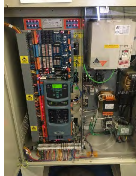
Torrance Courthouse – New Controller
