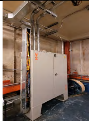
El Monte Courthouse – Elevator 5 New Controller
