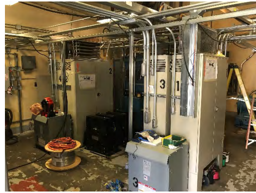
Beverly Hills Courthouse – New Elevators Controllers
