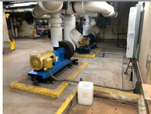
Van Nuys Courthouse East & West – Motors and VFDs
