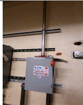
El Monte Courthouse – Elevator #5
