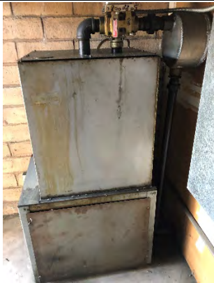
Walnut Creek Courthouse – Old Elevator Equipment
