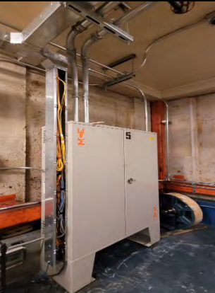
El Monte Courthouse – Elevator #5
