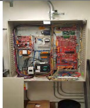
Northern Branch Courthouse – Elevator
