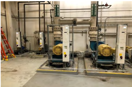
Van Nuys Courthouse East & West – Motors and VFDs
