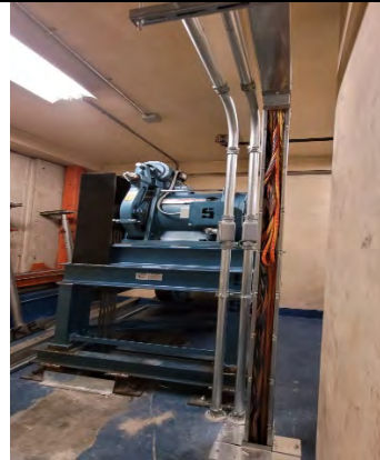
El Monte Courthouse – Elevator #5
