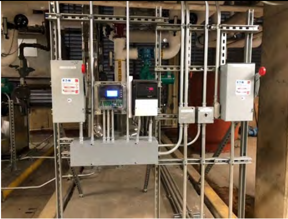
Van Nuys Courthouse East & West – New Controls
