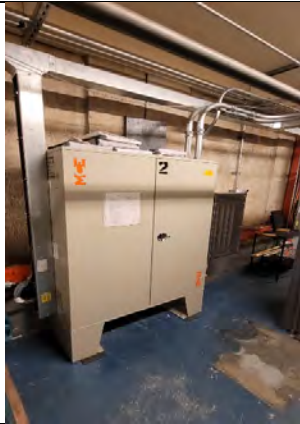
El Monte Courthouse – Elevator #2
