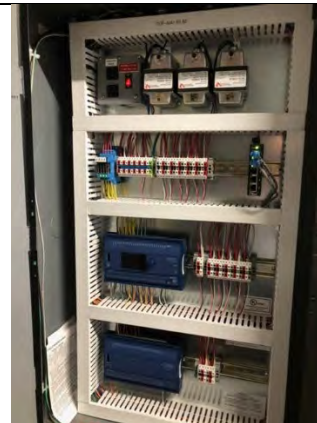
Van Nuys Courthouse East & West – New Controls
