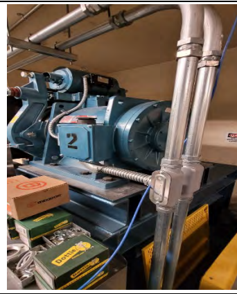
El Monte Courthouse – Elevator #2
