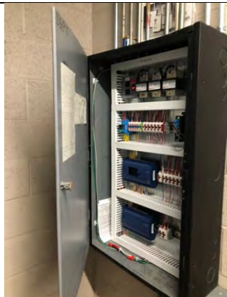
Van Nuys Courthouse East & West – New Controls
