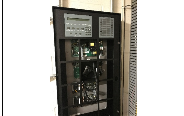
Carol Miller Justice Center Court Facility – Fire Protection
