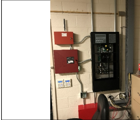
Carol Miller Justice Center Court Facility – Fire Protection
