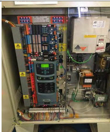
Torrance Courthouse Elevator Modernization – Controller After
