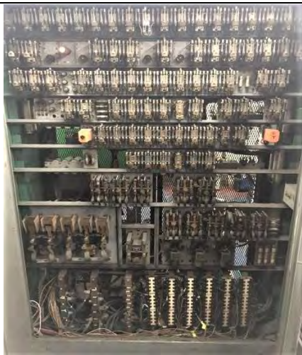
Torrance Courthouse Elevator Modernization – Controller Before
