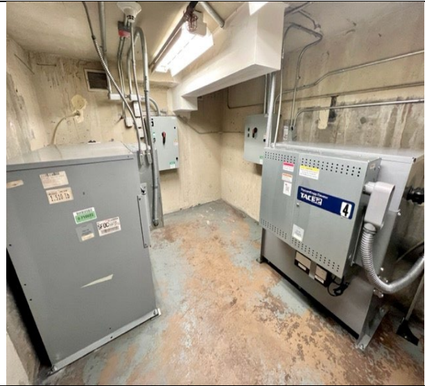
Hayward Hall of Justice - Elevator
