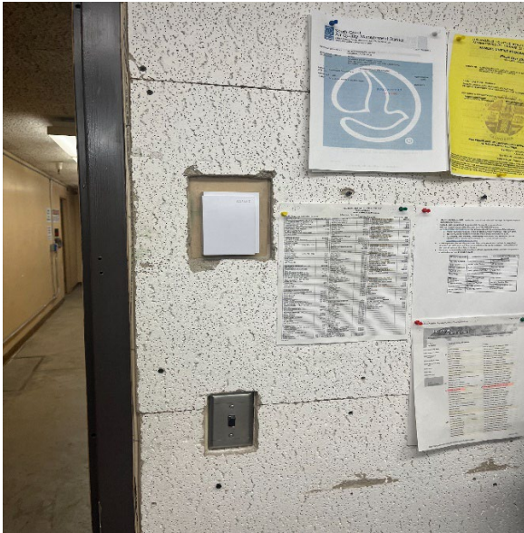
Alhambra Courthouse – BMS
