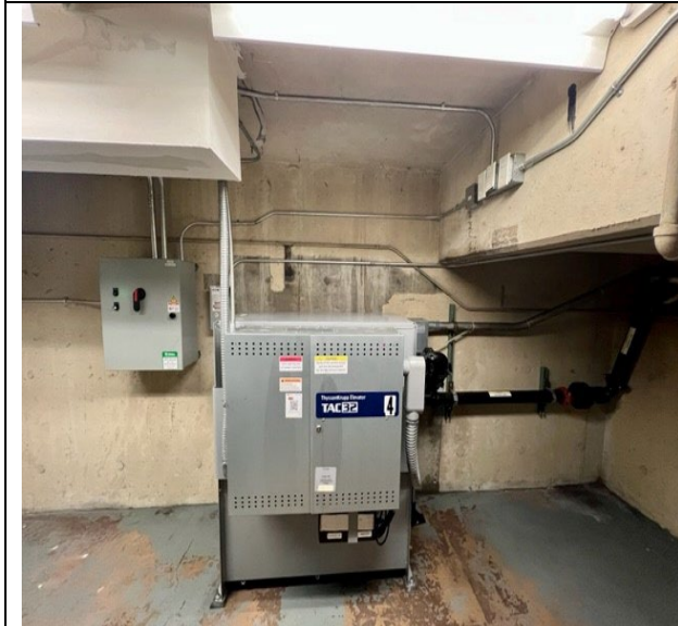
Hayward Hall of Justice - Elevator
