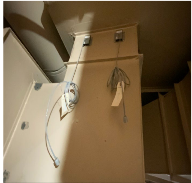
Alhambra Courthouse – BMS
