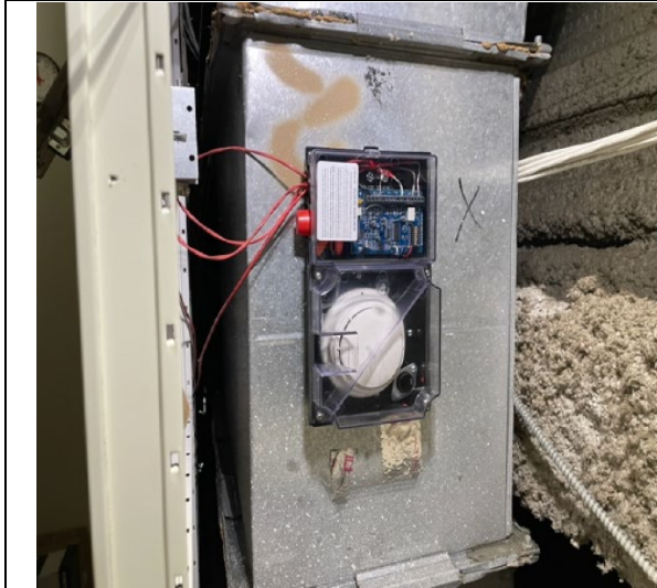
Betty Lou Lamoreaux Justice Center – Fire Alarm
