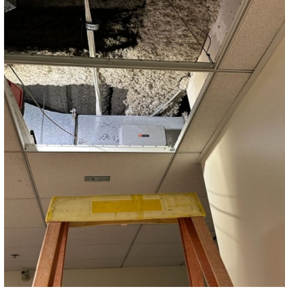
Betty Lou Lamoreaux Justice Center – Fire Alarm
