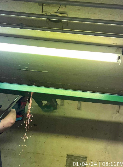
Hayward Hall of Justice – Elevator
