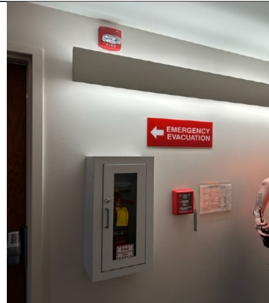
Betty Lou Lamoreaux Justice Center – Fire Alarm
