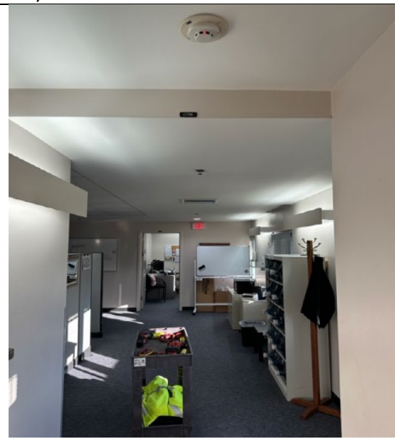
Betty Lou Lamoreaux Justice Center – Fire Alarm
