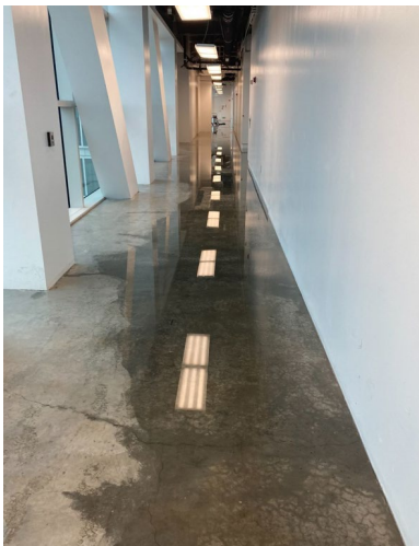
Interior flooding of the building from failure in helipad roof drainage system
