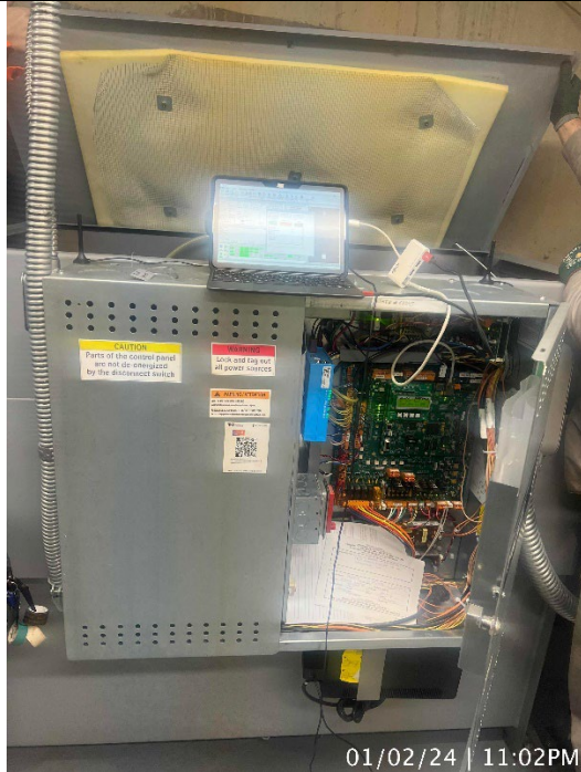
Hayward Hall of Justice – Elevator
