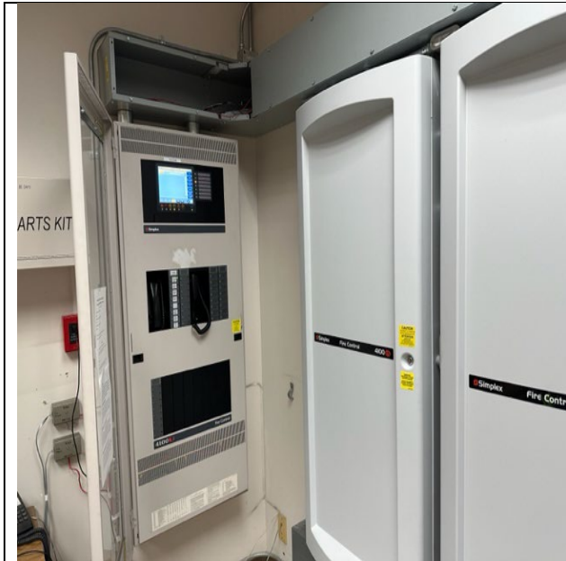
Betty Lou Lamoreaux Justice Center – Fire Alarm
