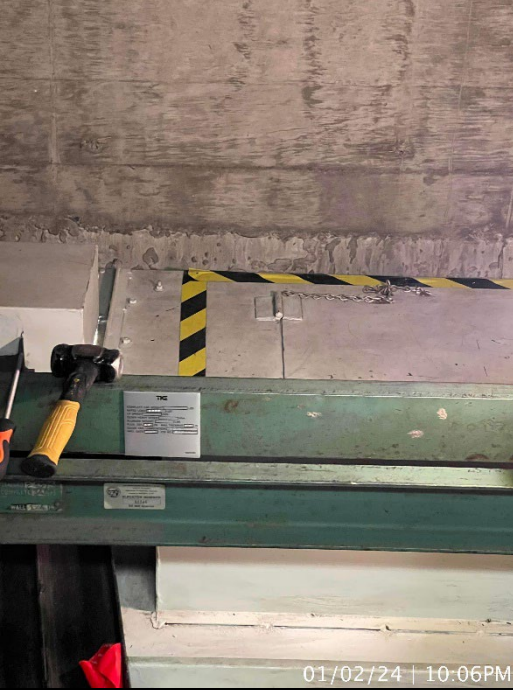
Hayward Hall of Justice – Elevator
