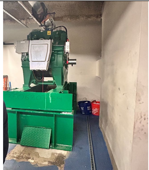
East Los Angeles Courthouse - Elevators
