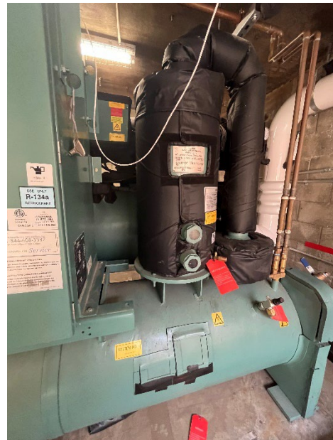
West Justice Center - Chiller
