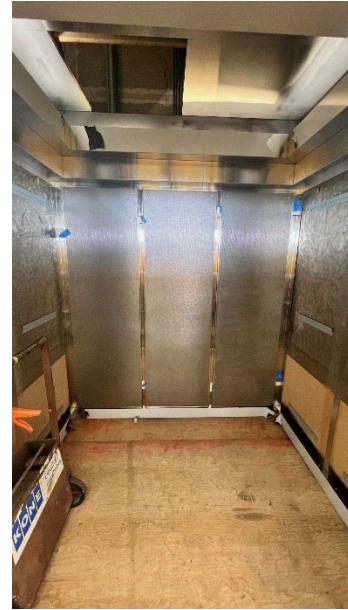
East Los Angeles Courthouse - Elevators
