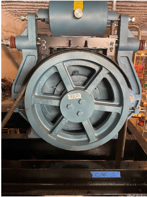
Civic Center Courthouse - Elevators
