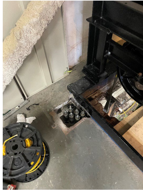
Civic Center Courthouse - Elevators
