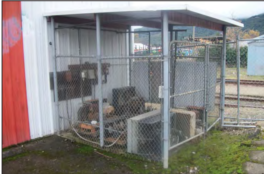
Air compressor and equipment storage enclosure on north side of Warehouse Building. View to the west.
