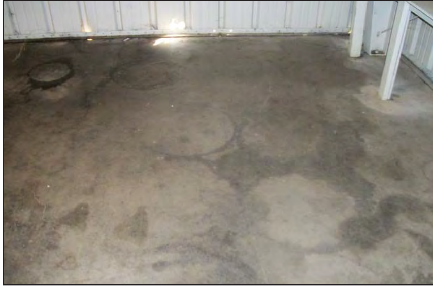
Probably Drum Staining on Cement in SW Corner of Shop Bldg. View to the south.
